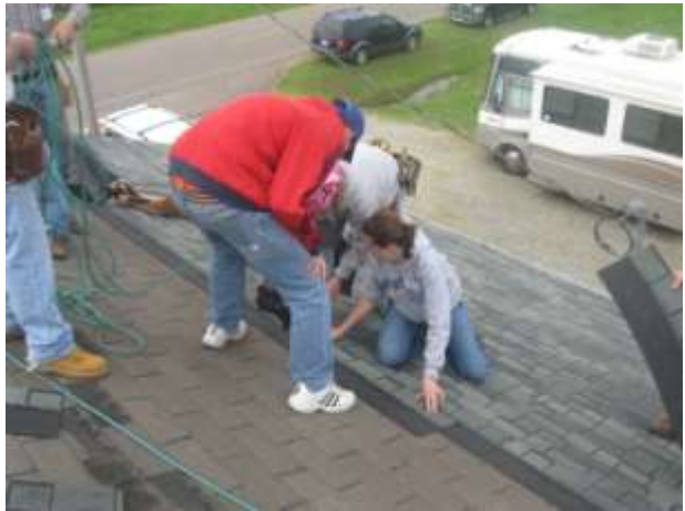
“Gunner” Derek nails the shingles while the “Alignment Sisters” make sure they are properly placed.
