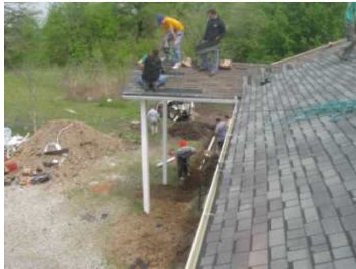
Roofing team installing shingles while the ground crew works on installation of the new septic tank.
