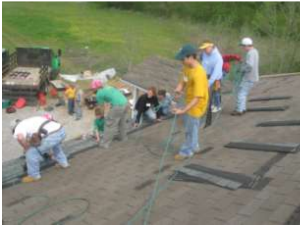
“Fast Eddie” moves the pneumatic hose out of the way while others continue placing shingles.
